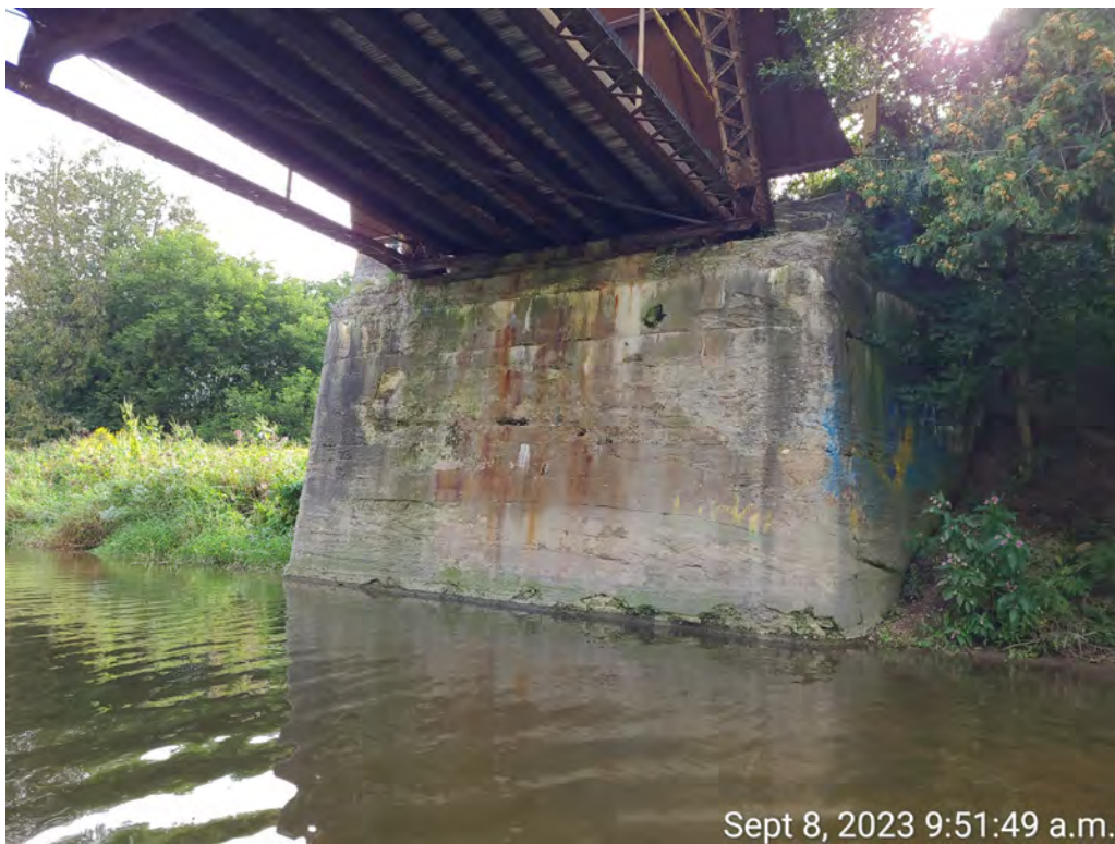
Photograph 16: East abutment showing light to severe erosion, spalling and disintegration
