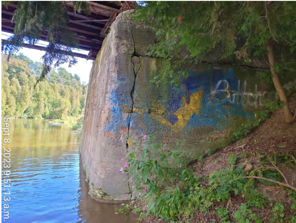
Photograph 17: East abutment, south wingwall showing wide vertical crack at wingwall/abutment interface and wide horizontal crack at cold joint.
