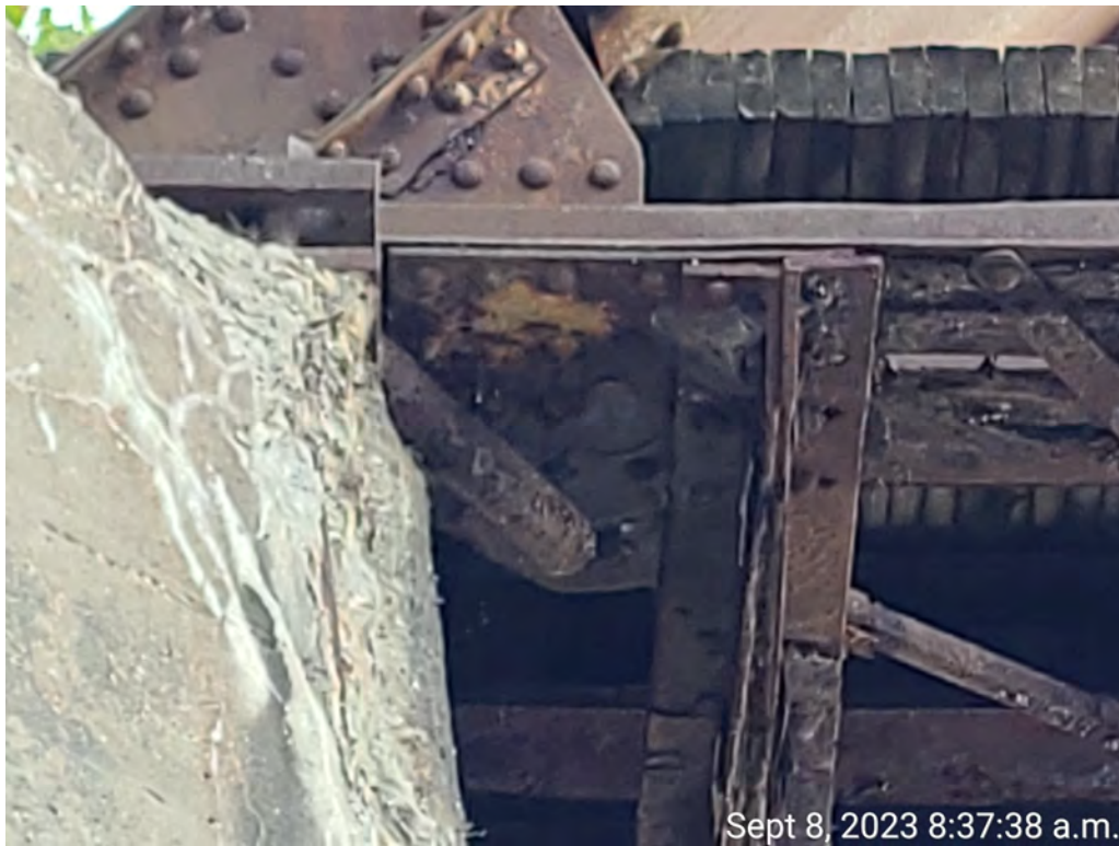
Photograph 9: West abutment, south bearing showing dislodged bearing roller pin.
