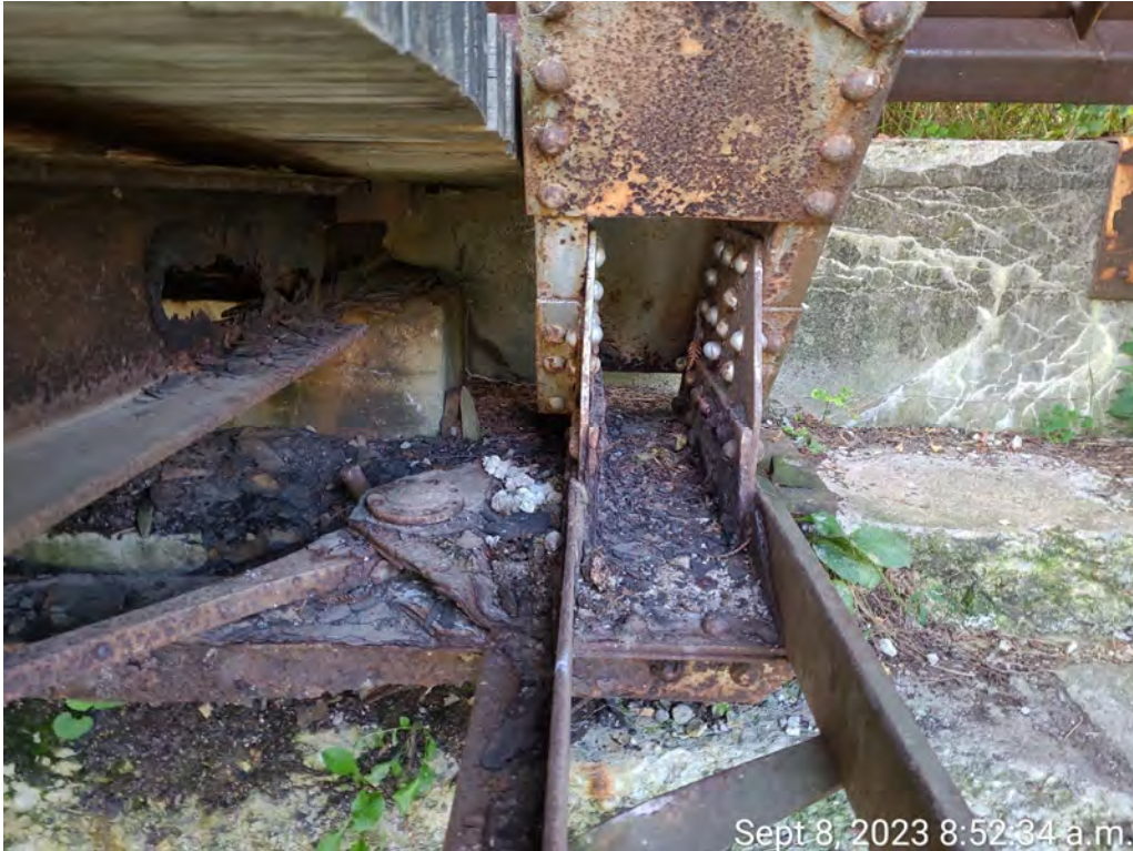
Photograph 2: Stringer in Bay 1 and east abutment, south bearing. Note complete loss of section in stringer web and loss of contact between wood deck and stringer top flange.
