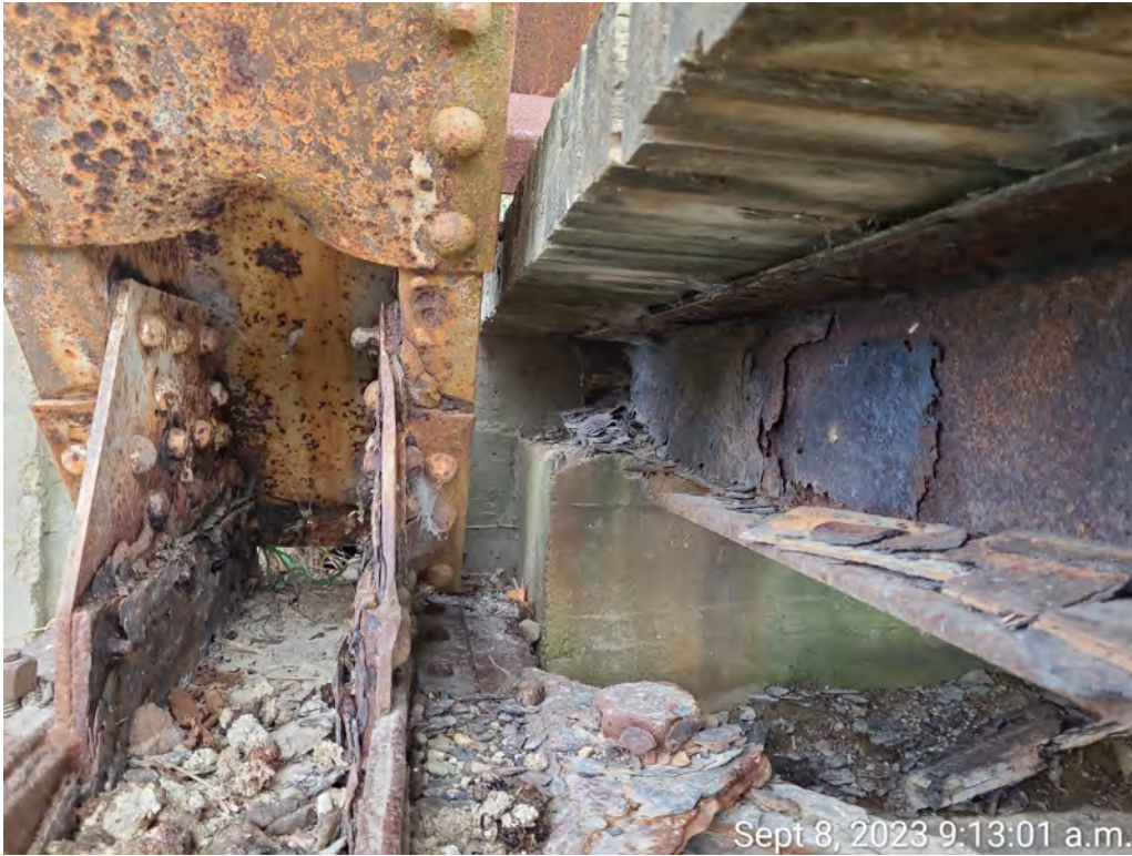
Photograph 3: Stringer in Bay 9 and west abutment, south bearing. Note complete loss of section in stringer bottom flange at stringer bearing seat, severe corrosion of bearing plates and severe corrosion of bottom lateral.
