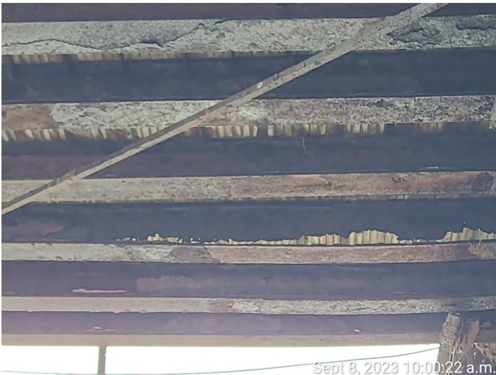
Photograph 4: Stringers in Bay 1 looking north. Note complete loss of section in stringer webs.
