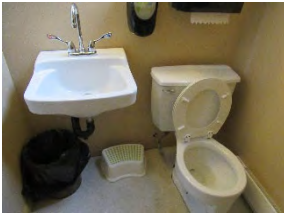
8 SJL - lower level washroom toilet and sink
