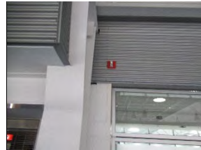
17 WMC 2nd Floor Arena visual alarm
