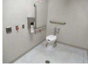
3 HCC - washroom toilet area
