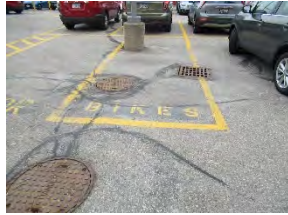
30 WAO Accessible parking aisle
