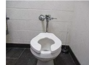
20 WAO Basement - unisex washroom - no grab bars
