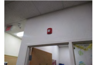
14 WAO office area - visual alarm
